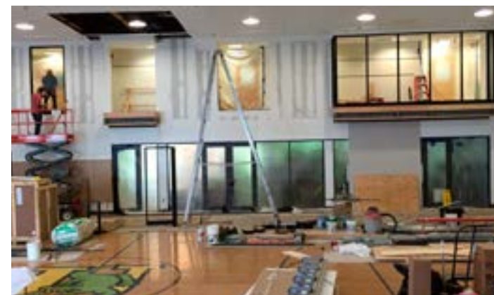
The frames for the bump-out windows and third and fourth grade reading nooks are installed and awaiting glass.
