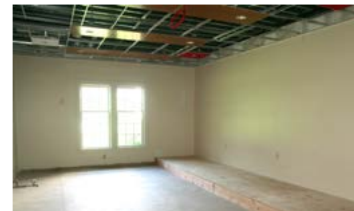
The complete renovation of the instrumental classroom is almost done and includes a riser for guitar ensemble.
