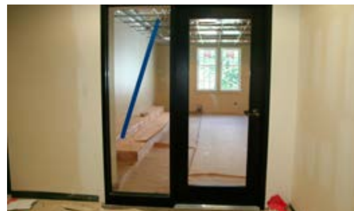
The new second floor performing arts classroom is taking shape with built-in choral risers and a mirrored wall with ballet barre.
