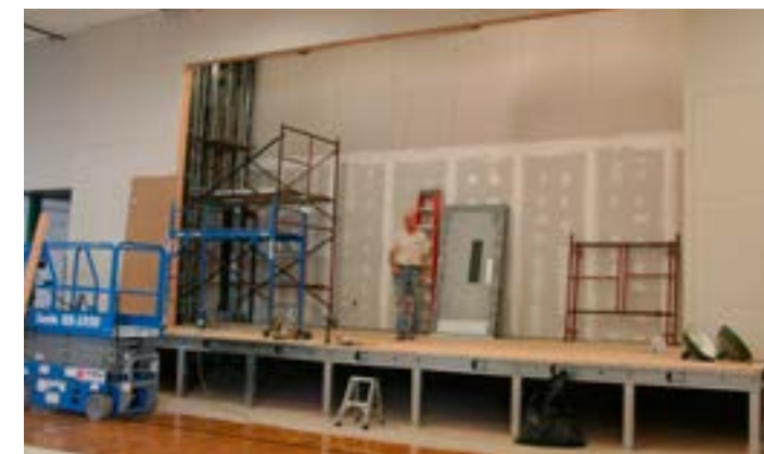
The temporary wall is down and framing is almost complete on the new performing arts space and lift.
